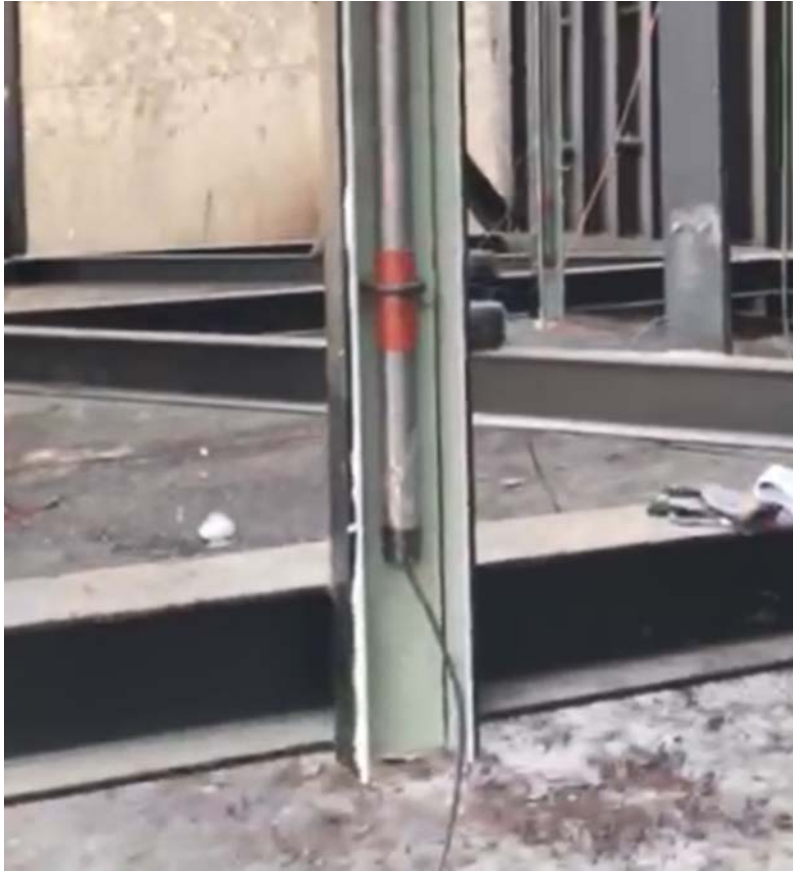
Figure 3. Screenshot from a video that shows the bottom of the cast iron tubular anode string mounted in one of the channels on the frame side of Gate 4. The screenshot shows that the cable lead is present at the bottom of the anode string. The anodes are mounted using coated U-bolts and a fiberglass isolation panel (red). The fiberglass bonded to the interior of the channel is present, and cured epoxy (white) can be seen where the fiberglass joins to the steel channel.
