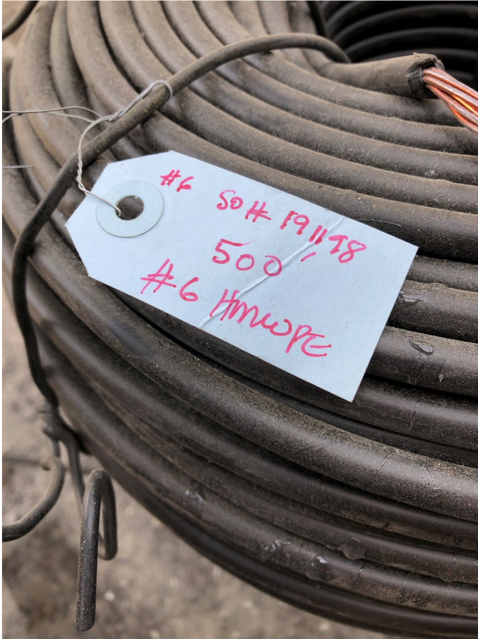
Figure 4. Identifying tag on anode cable lead bundle showing a 500-ft length. The cable bundle was measured, and it was confirmed that each anode lead was 500 ft long instead of the 250-ft length specified
