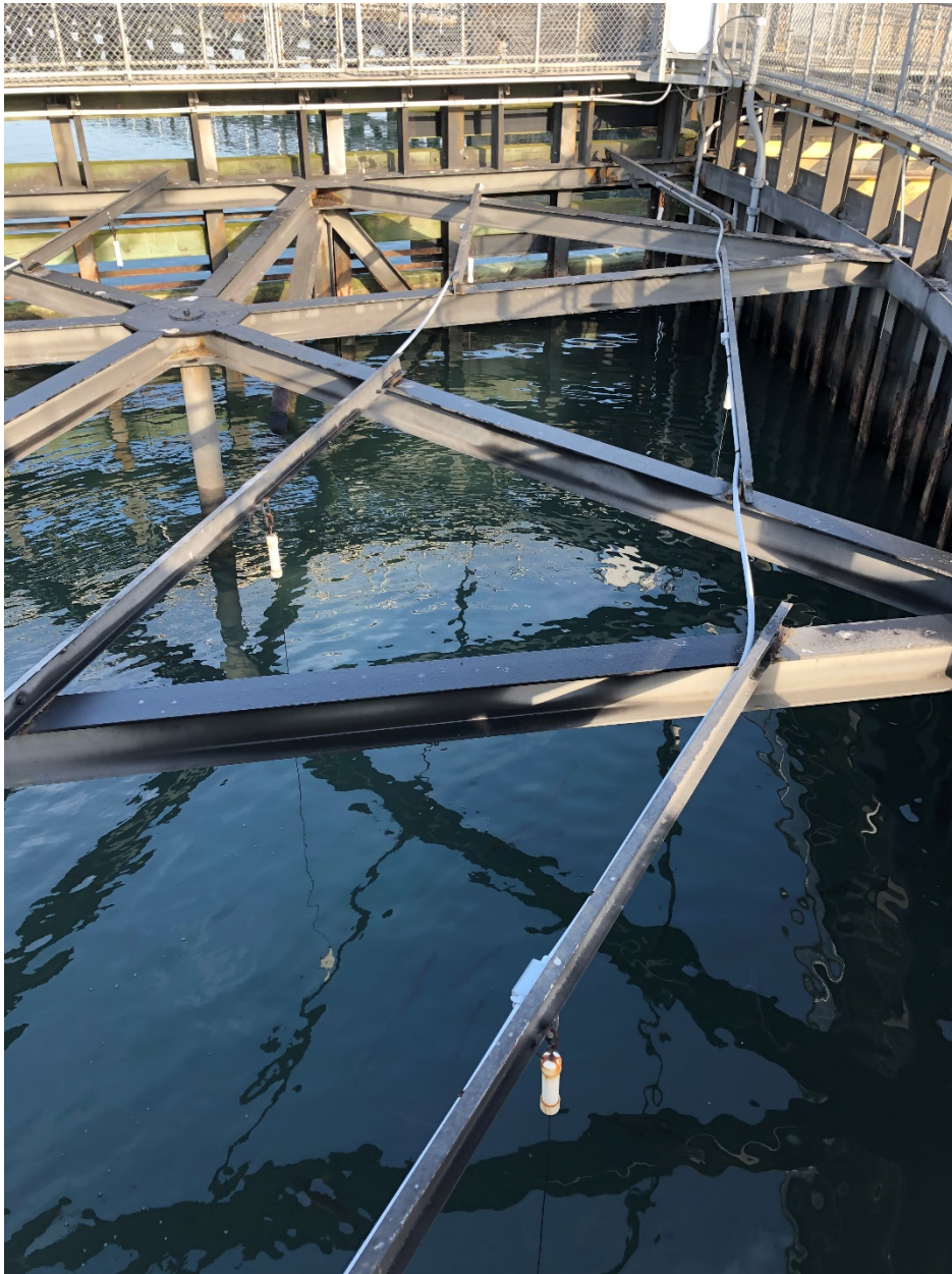
Figure 1. Conduit on the frame side of Gate 1 (east gates). Some conduit is running over open water rather than following structural members. MMO anode wires remaining from the previous CP system are seen hanging into the water. Concrete anchors keep the wire anodes in position.
