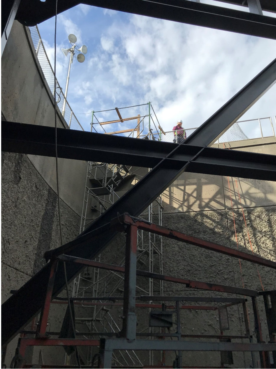
Figure 7. View from the pit of Gate 4. A manlift and structural frame members can be seen in the foreground. In the background, Vince Hock (USACE ERDC-CERL) can be seen standing at ground level by the edge of the pit.
