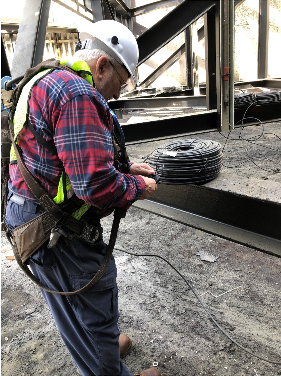
Figure 5. Vincent Hock (USACE ERDC-CERL) labelling the anode lead based on the design drawing for identification purposes after pulling the cable through the conduit.
