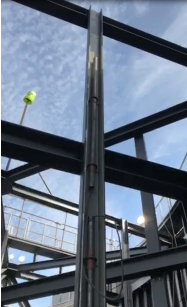
Figure 2. A screenshot from a video that shows the cast iron tubular anode string mounted in a channel on the frame side of Gate 4. The cable lead at the top of the string is not present. The bond between the two cast iron anodes is 4 ft instead of 1 ft, so the cable does not fit between the anodes as it should. The proposed solution is to coil the cable and fit the coil within the channel. Also shown is the fiberglass bonded to the interior of the channel. This prevents over-polarization of the metal where the anodes are mounted. Instead, the cathodic current will polarize the frame pieces and channel across from each anode pair.
